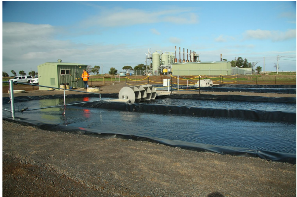
Fig. 1 Two high rate algal ponds at Melbourne Water Western Treatment Plant, Australia designed by the authors and fed anaerobic and facultative lagoon treated domestic wastewater
